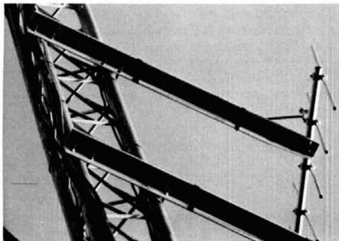
Antenna-mounting hardware consists of stainless steel and heavy-gauge aluminum.
